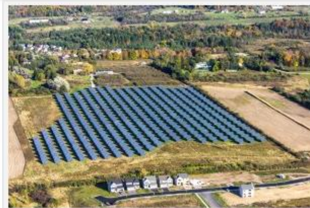
366 solar trackers and 8,784 JA Solar modules at Claire Solar in So. Burlington, Vt., the largest solar installation of its kind in North America
