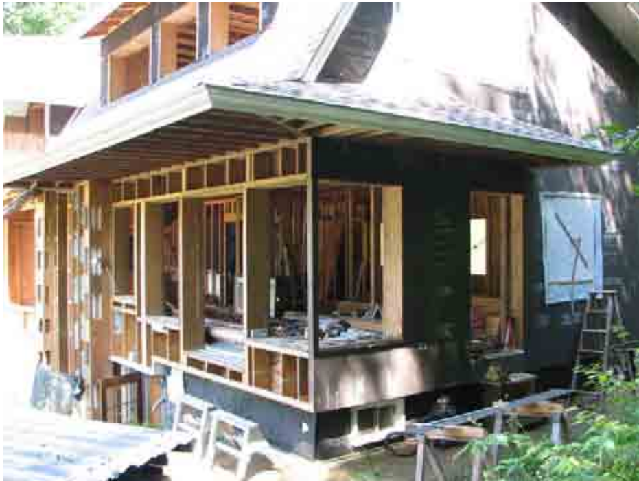
16" thick Larsen truss walls, 26 years off grid. both energy reduction and energy production
