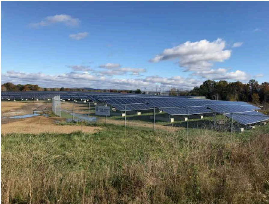
South Burlington Landfill, South Burlington, VT – 2.1MWp
